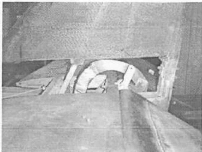
General composition of the Teate KR internal elevator balance system. Cast lead counterbalance weight is taped into position on curved aluminum arm.
